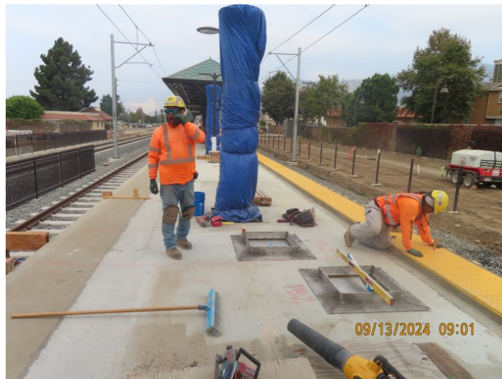
Glendora Station - Pill box paver covers
