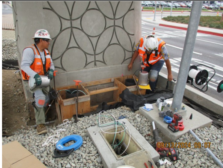
Lone Hill - Bridge lighting
