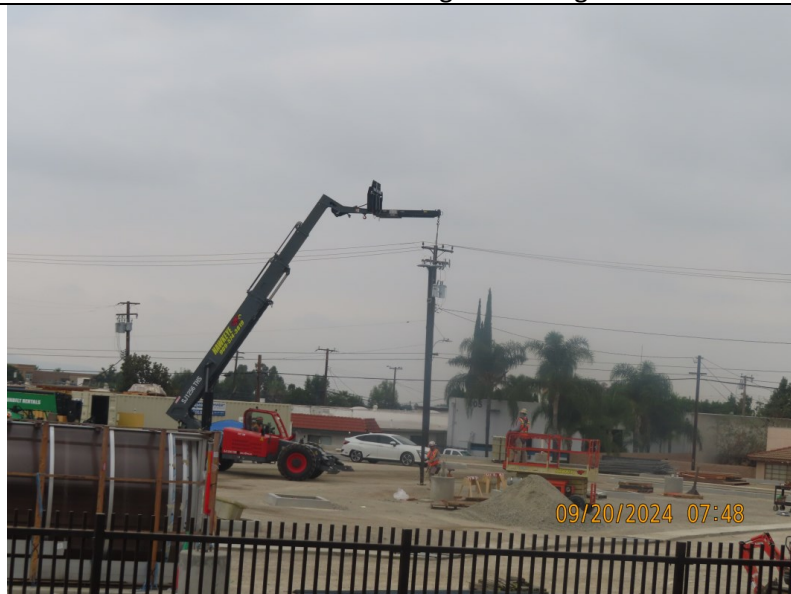
Glendora Station Parking - Light poles
