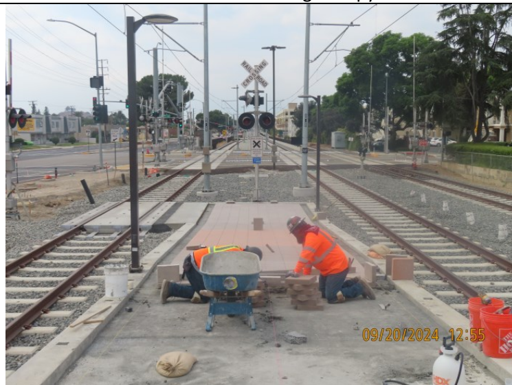
Pomona Station - Electrical wiring
