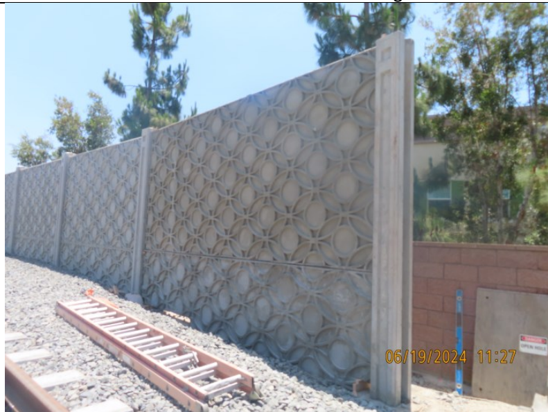
San Dimas/Walnut - Soundwall panel
