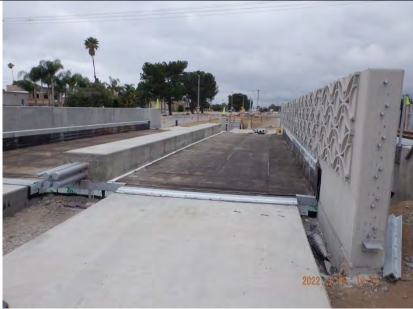
Live Oak—Ductbank encased
