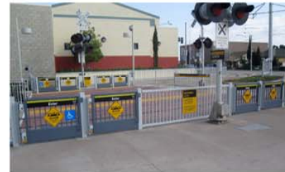
Pedestrian Grade Crossing Gates and Flabbers
