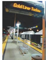
Variable Message Sign (VMS)
