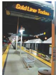
Variable Message Sign (VMS)
