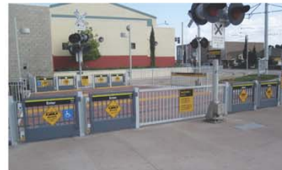
Pedestrian Grade Crossing Gates and Flashers
