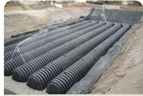
The stormwater management system captures the first 112,000 gallons of rain water; removes contaminants before traveling to subterranean chambers that will slowly release water into the groundwater aquifer.
