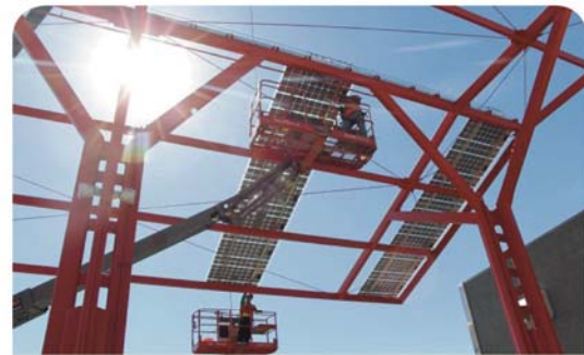
Using cranes, workers placed 714 individual solar panels that will create nearly 22,000 kilowatt hours per month of electricity.
